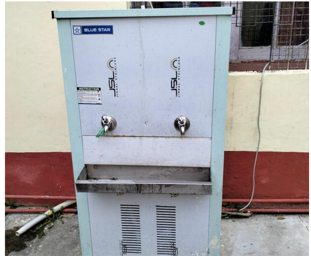
Push taps installed for water conservation
